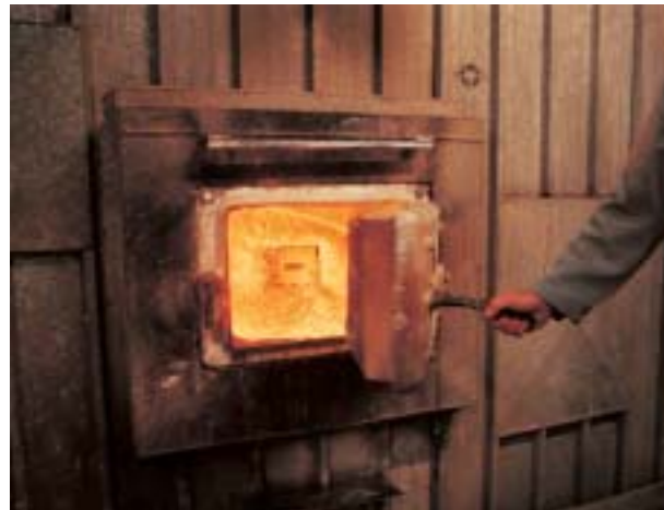
Co-generation plant at Mainz coffee factory, Germany, where spent coffee grounds are used as fuel
