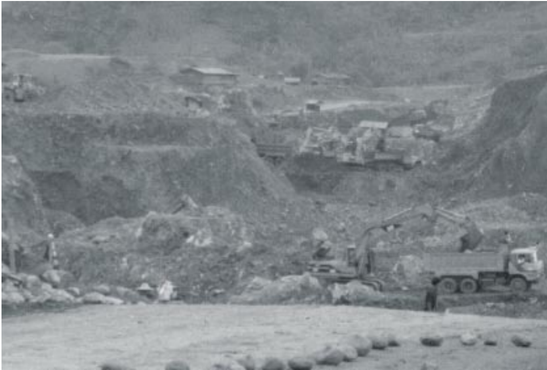
Heavy duty equipment working at Hpakant gem mine, Kachin State (Credit: Images Asia)
